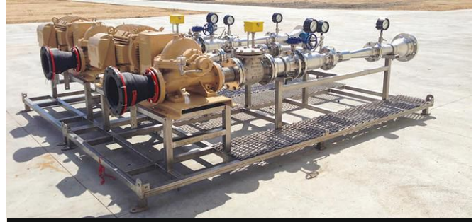
Image 1. Platform-mounted injector systems aerate water in the Hickory Aquifer Groundwater Treatment Facility in San Angelo, Texas, to remove dissolved iron. Shown are two of the four sidestream aeration systems. (Images courtesy of Mazzei)
