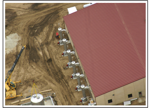
Aerial view of the DS1600 LFs and the AOP building during construction.
